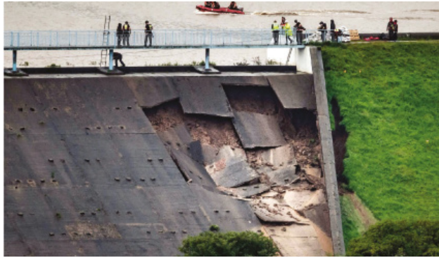
The Final Stage of Collapse of Panels. Note the undermining of the left-hand chute wall Photo: Balmforth Report
