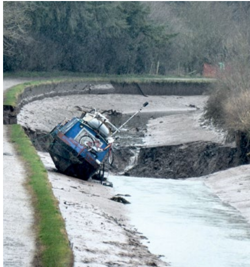
The Middlewich breach Photo Harry Arnold, Waterway Images
