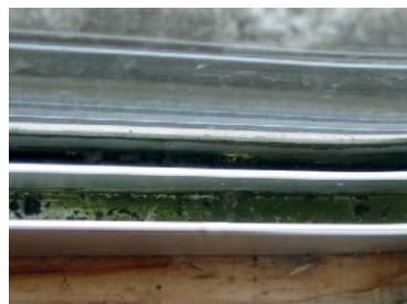
Window channel with a year's growth of moss
