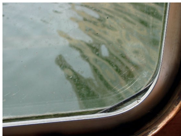
Misplaced window sealing cord
