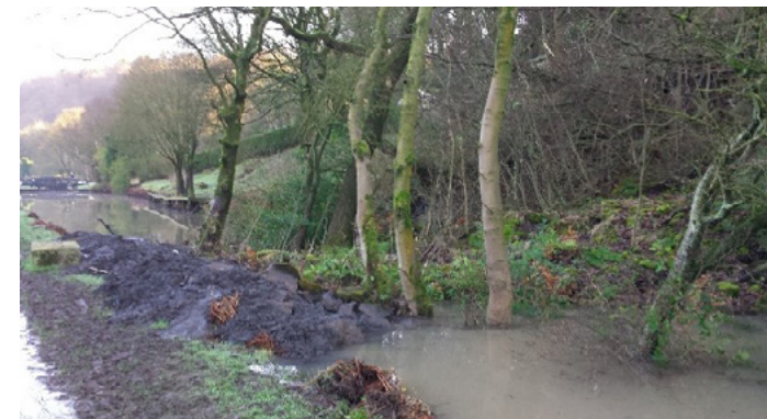
A collapsed embankment on the Rochdale Canal
