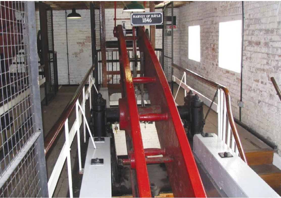
Harvey engine beam weighing 4½ tons in Crofton Pumping Station Photo: Derek Carvin www.gypsyover.co.nz
