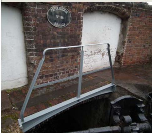
New rails on a lock tail bridge at Penkridge as reported last issue.
