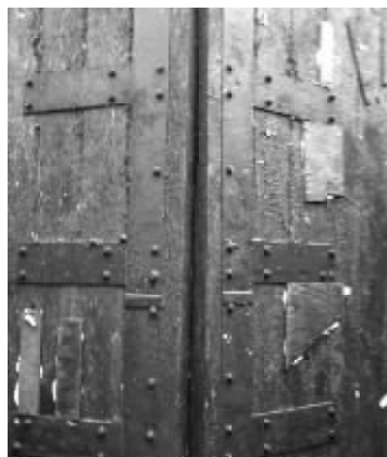
Ply and foam patched lock gate
